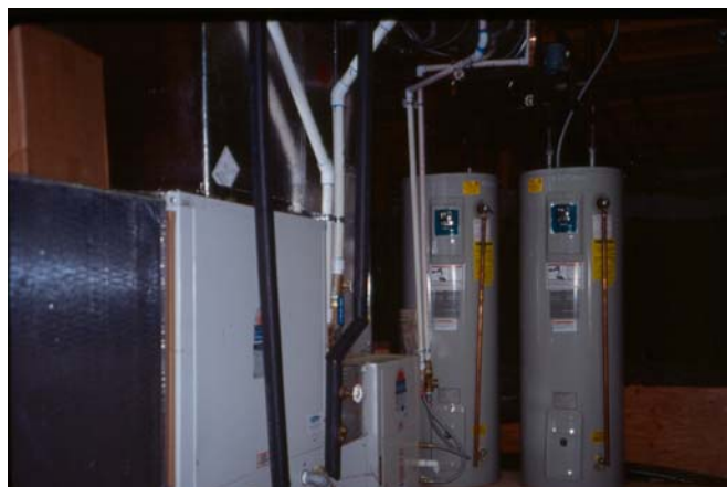
Figure 3. Water to water heat pump.
