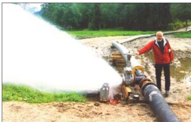
Dick Benoit venting the main geothermal supply line to the power plant.
