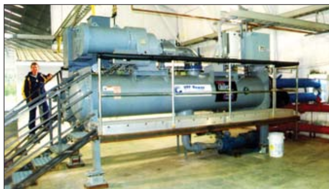
The 200kW United Technologies power plant.
