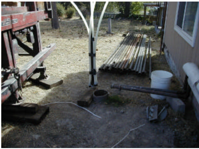
Figure 7. PEX DHE prior to installation, showing the two PEX U-tubes fastened to the steel pipe from the old DHE, which was used as an installation guide, anchor and convection promoter.
