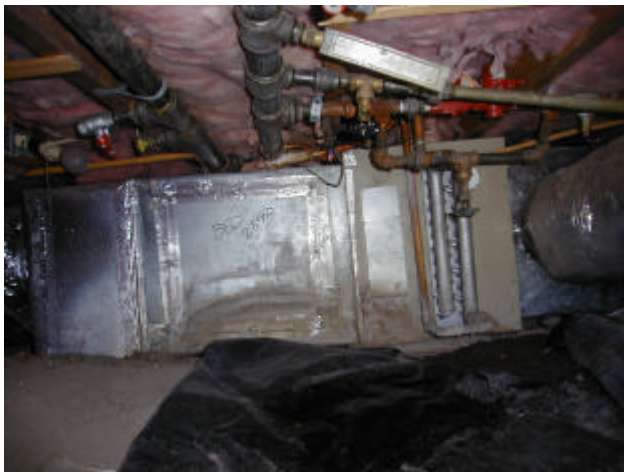
Figure 3. Air-handling unit with hot water coil installed in the crawl space.
